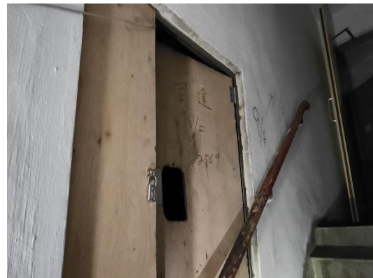
Photo 4-1 (d): Staircase Landing of 10/F, Wang Kin House (Photo Taken After the Fire)
