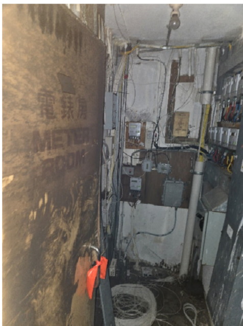
Meter Room Overview (Photo M1)
