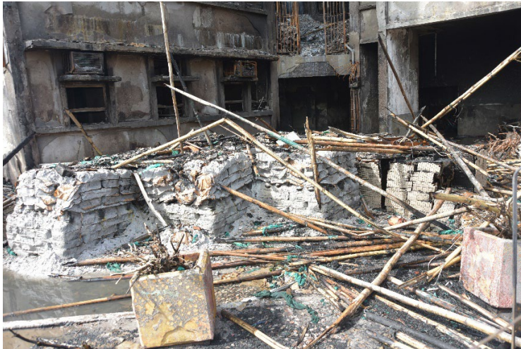
Photo 4-9 (c): Post-Fire Condition outside the East Re-entrant of Wang Cheong House
