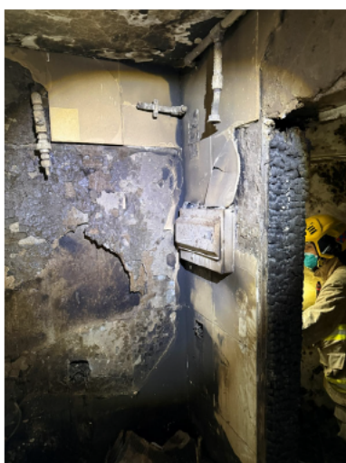
Distribution Board in Kitchen of Flat 105 (Photo B3)
