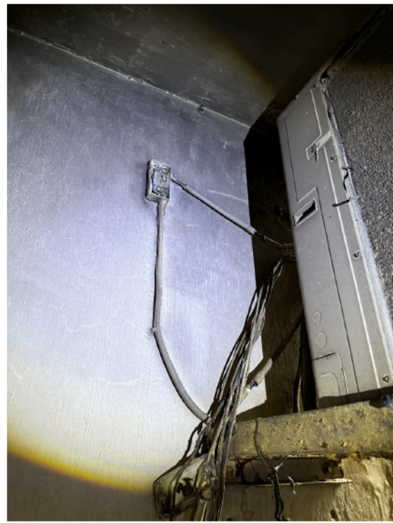
Air Conditioner in Bicycle Parking Space (Photo G6)
