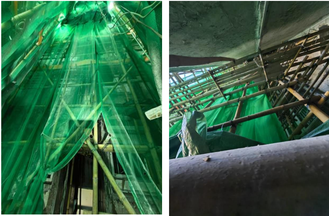
Photos 6-6 (a) & (b): Continuous Fuel Source in the Re-Entrant
