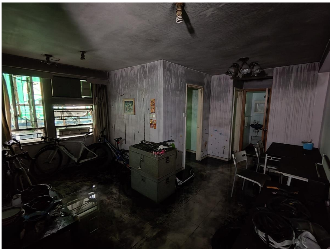
Photo 8-3 (b): Unit Sustained Severe Damage – Flat 01, Wang Yan House
