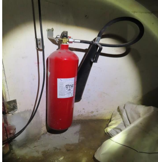
Photo showing the Fire Extinguisher in FS pump room on G/F Wang Chi House (Photo taken on 1.12.2025)
