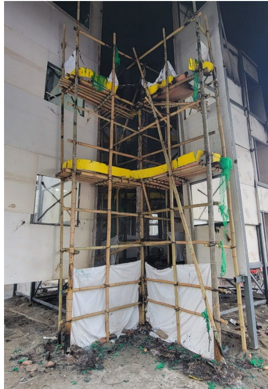
Photo 2-16 (n): Post-Fire Condition in Test 12 [Sample 4 (Wang Chi House)]
