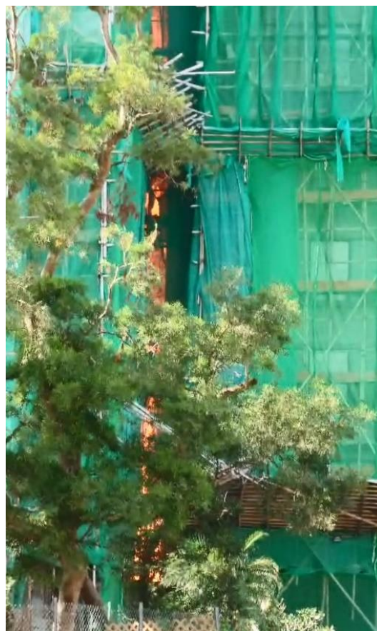
Photo 5-4: Fire Spread to About 8/F at About 1457 Hours
