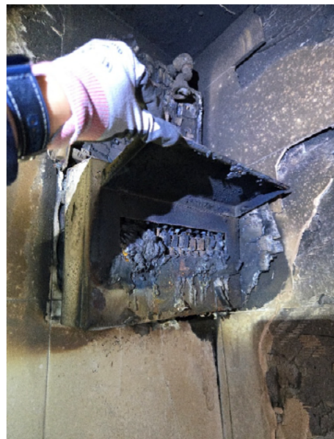
Interior of Distribution Board in Kitchen of Flat 104 (Photo A4)
