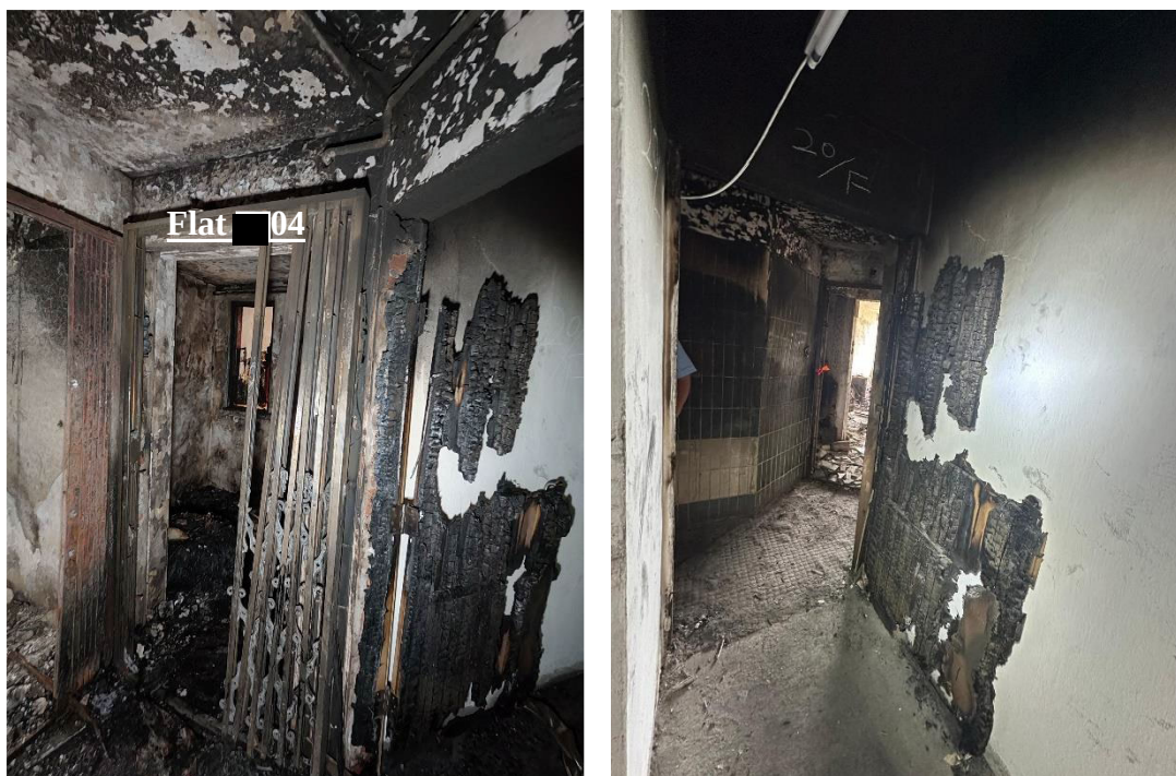
Photos 8-13 (e) & (f): Damaged Smoke Stop Door on [REDACTED]/F of Wang Yan House
