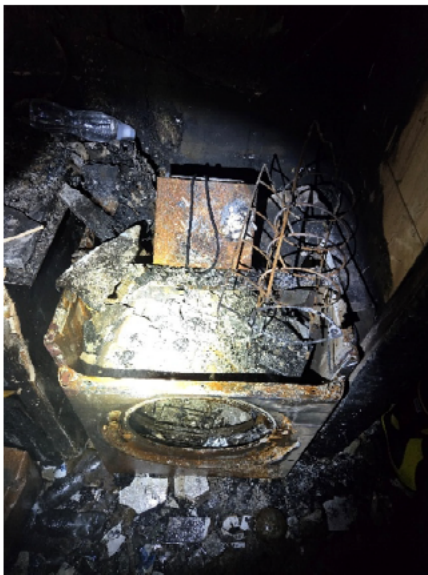
Washing Machine in Kitchen of Flat 104 (Photo B7)
