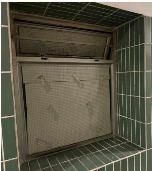
Photo 4-2 (b): Lift Lobby Window (Photo Taken After the Fire)
