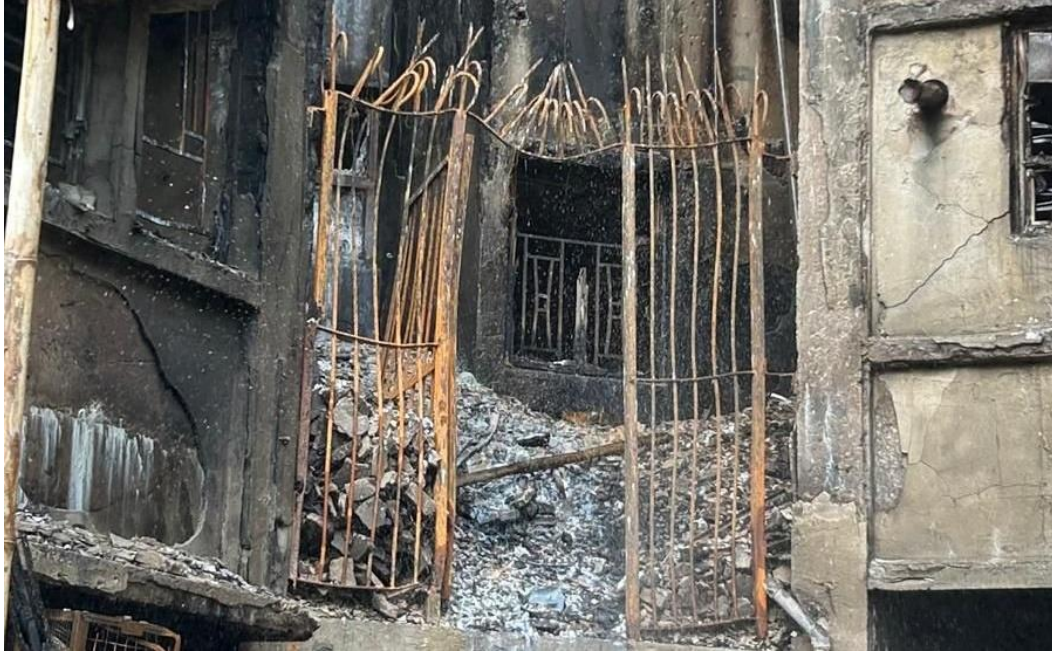
Photo 6-1: Debris Piled up on the Flat Roof Outside Flats 104 and 105 of Wang Cheong House
