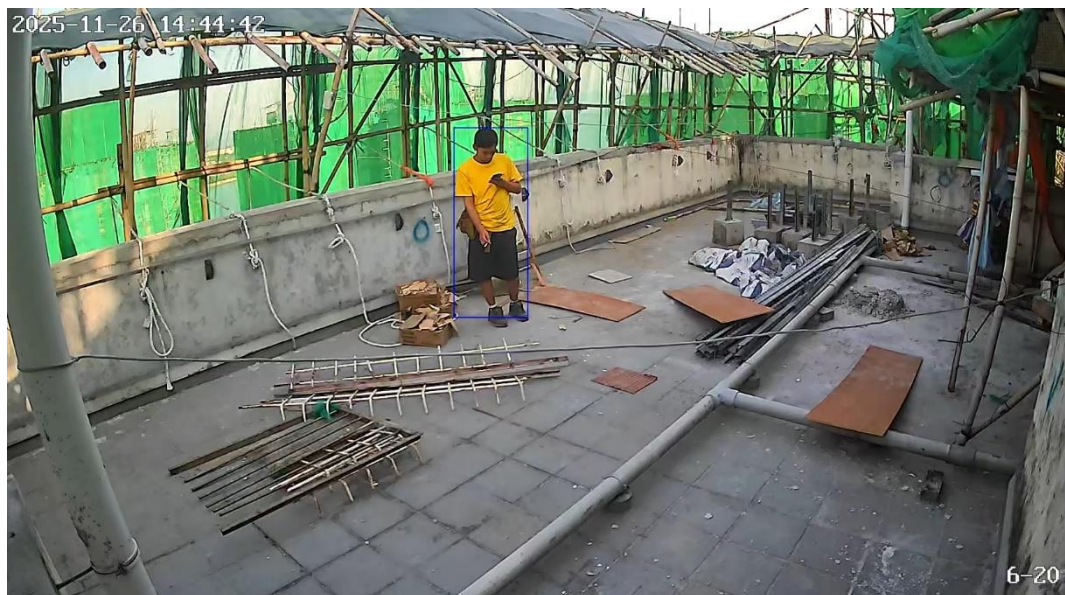
Photos 6-5 (e) & (f): Construction Workers Were Smoking on R/F of Wang Cheong House at About 1411 hours and 1445 Hours 66
