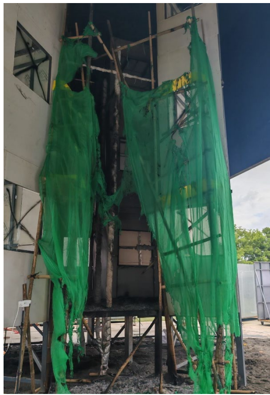
Photo 2-12 (d): Post-Fire Condition in Test 8 using non-FR Safety Nets
