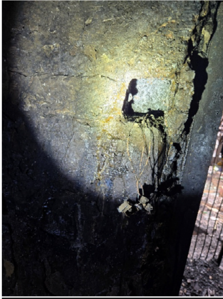
Socket Outlet in Kitchen of Flat 104 (Photo A5)
