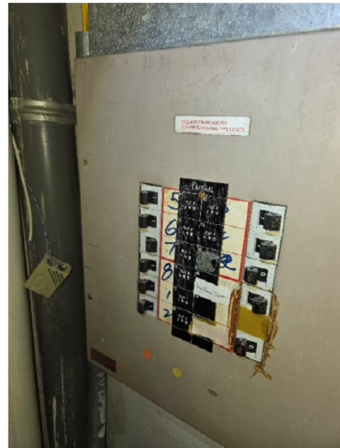
Distribution Board for Different Flats in Meter Room (Photo M4)
