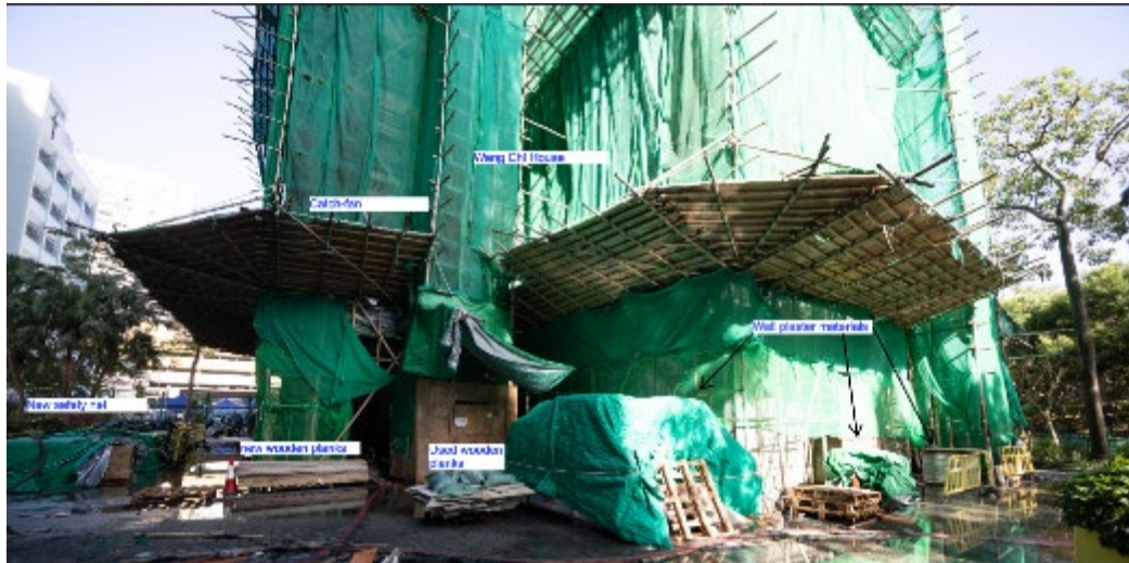
Photo: combustible materials outside Wang Chi House
