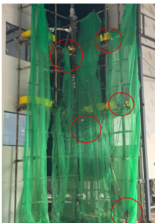
Photo 2-1 (b): Fire Spread along Uncertified Safety Nets
