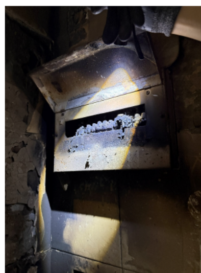
Interior of Distribution Board in Kitchen of Flat 105
