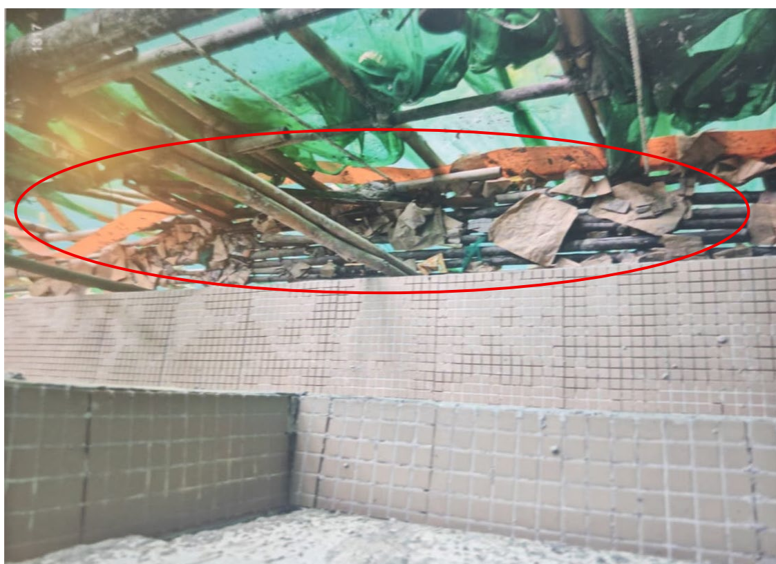
Photos 4-7 (c): Combustible materials on the External Scaffolding
