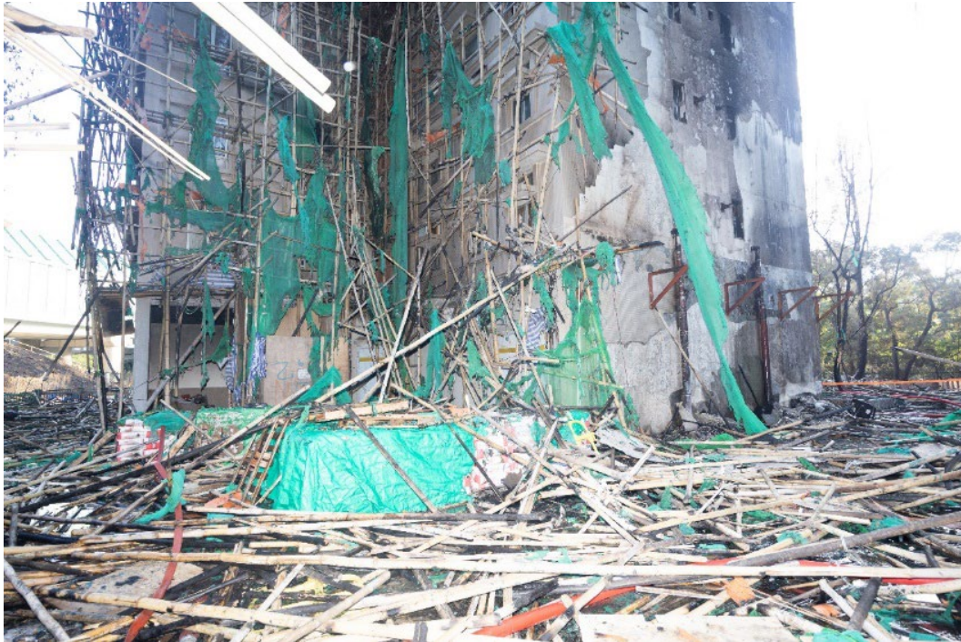
Photo 4-9 (h): Post-Fire Condition outside the North Re-entrant of Wang Cheong House
