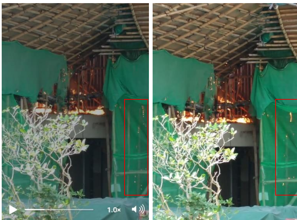
Photos 8-19 (a) & (b): Flaming Droplets Dripping From Burning Materials Observed During the Initial Stage of Fire
