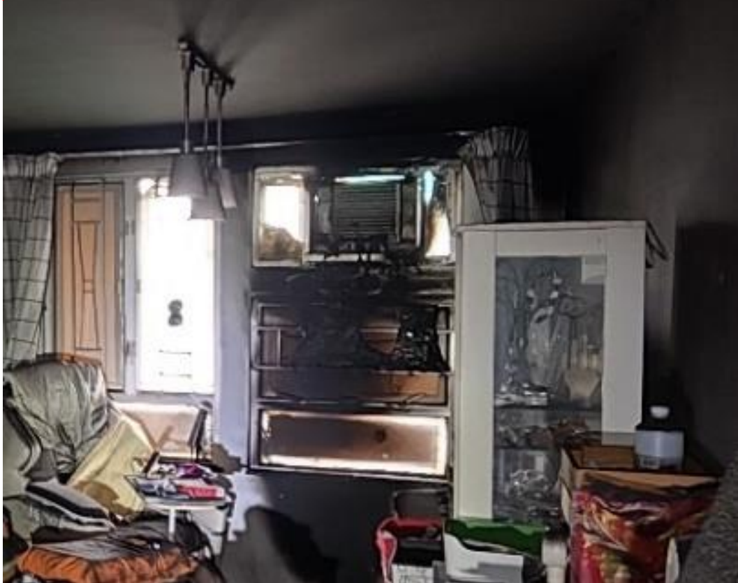
Photos 8-7 (a) & (b): Fire Spread Into Flat 08 via the Air-conditioner
