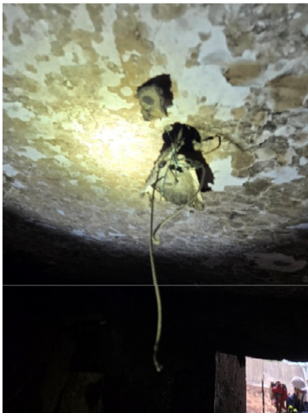
Ceiling Lighting in Kitchen of Flat 104 (Photo A7)
