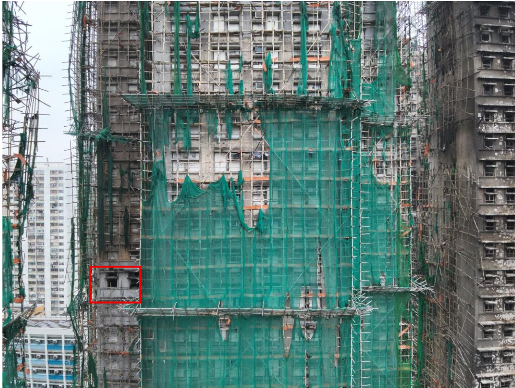
Photo 8-8 (g): External Post-Fire Condition of Flat ■ 02
