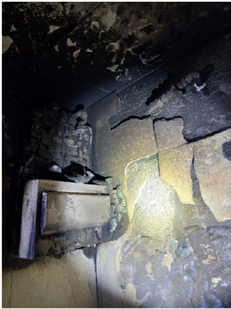
Distribution Board in Kitchen of Flat 104 (Photo A3)
