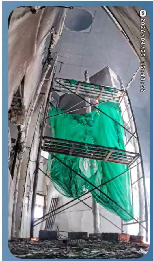
Photo 2-9 (d): Post-Fire Condition of Sample 4 (Wang Chi) (Fully Consumed)
