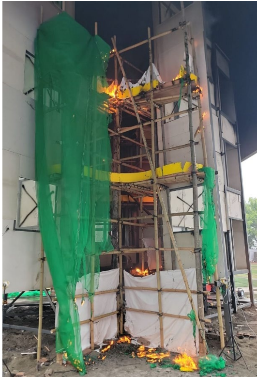
Photo 2-16 (m): Secondary Ignition in Test 12 [Sample 4 (Wang Chi House)] 36
