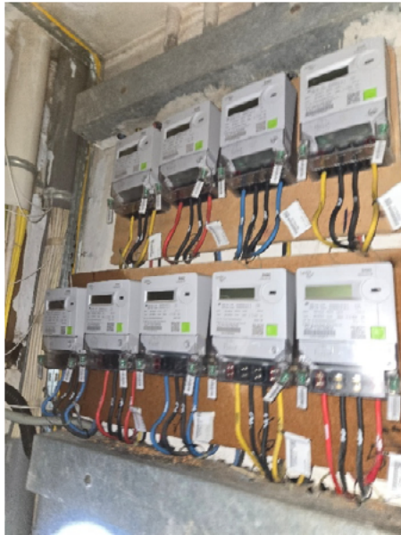
Electric Meters in Meter Room (Photo M3)
