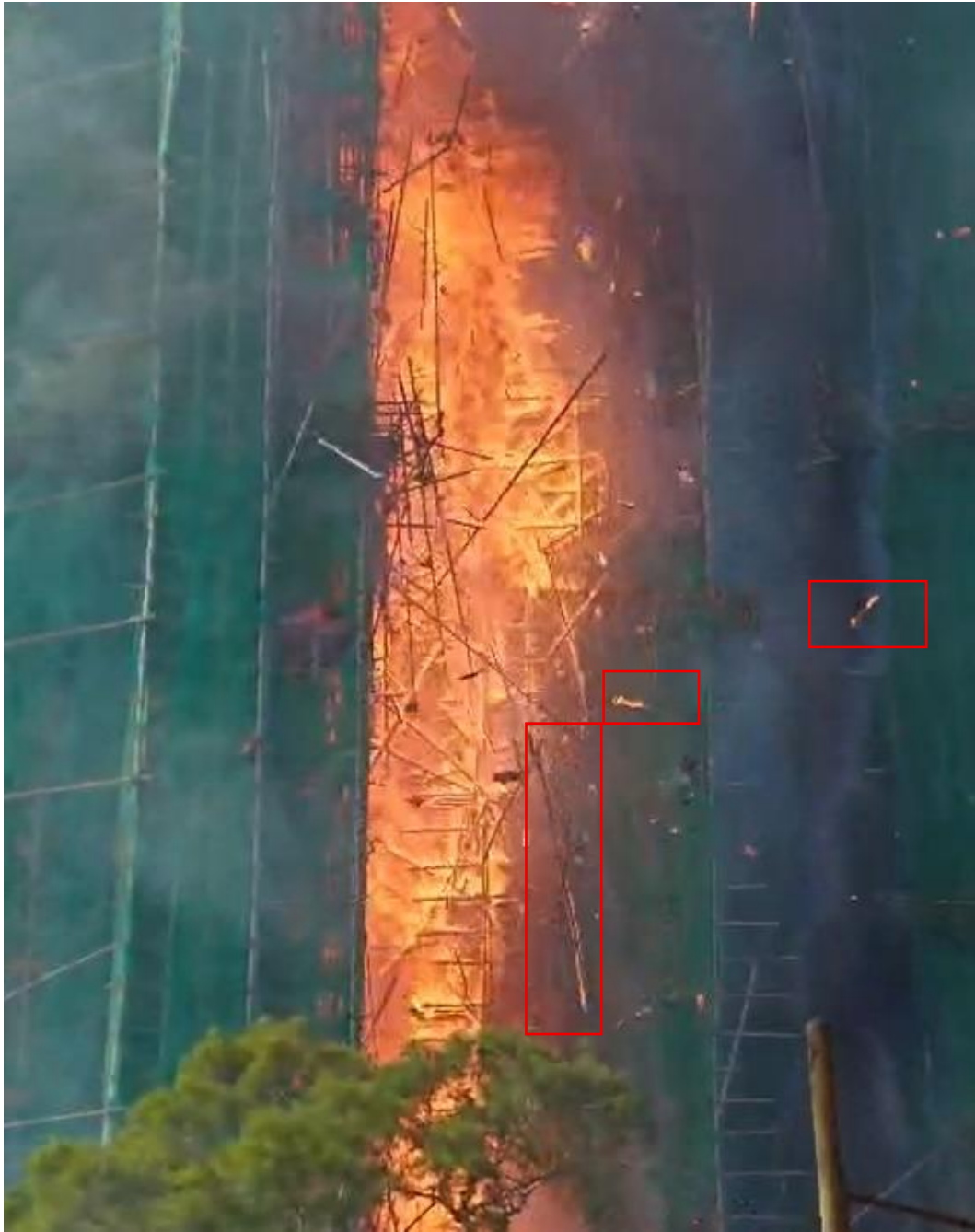
Photo 8-17: Collapsed Burning Debris From the Damaged Bamboo Scaffolding
