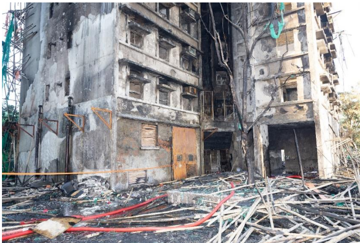
Photo 8-21 (e): Post-Fire Condition Outside the West Re-Entrant of Wang Cheong House
