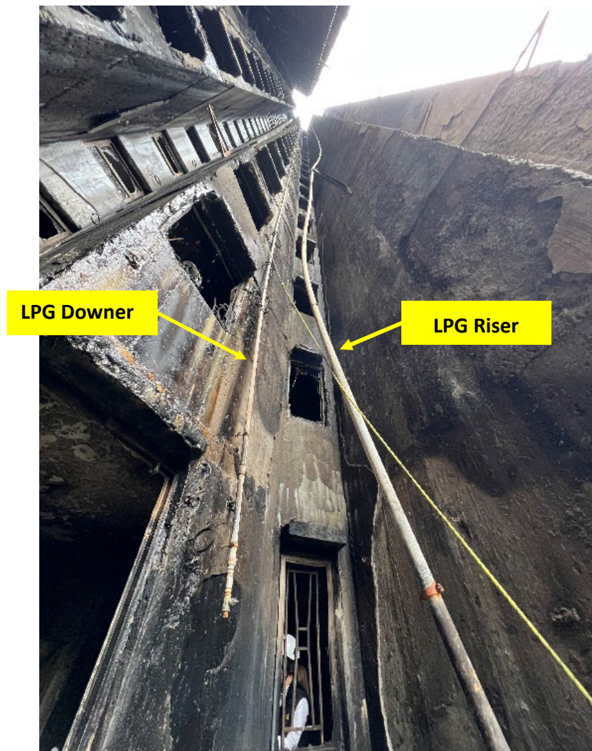
Photo 5 - Deformed LPG riser and downer at Wang Cheong House with no sign of rupture
