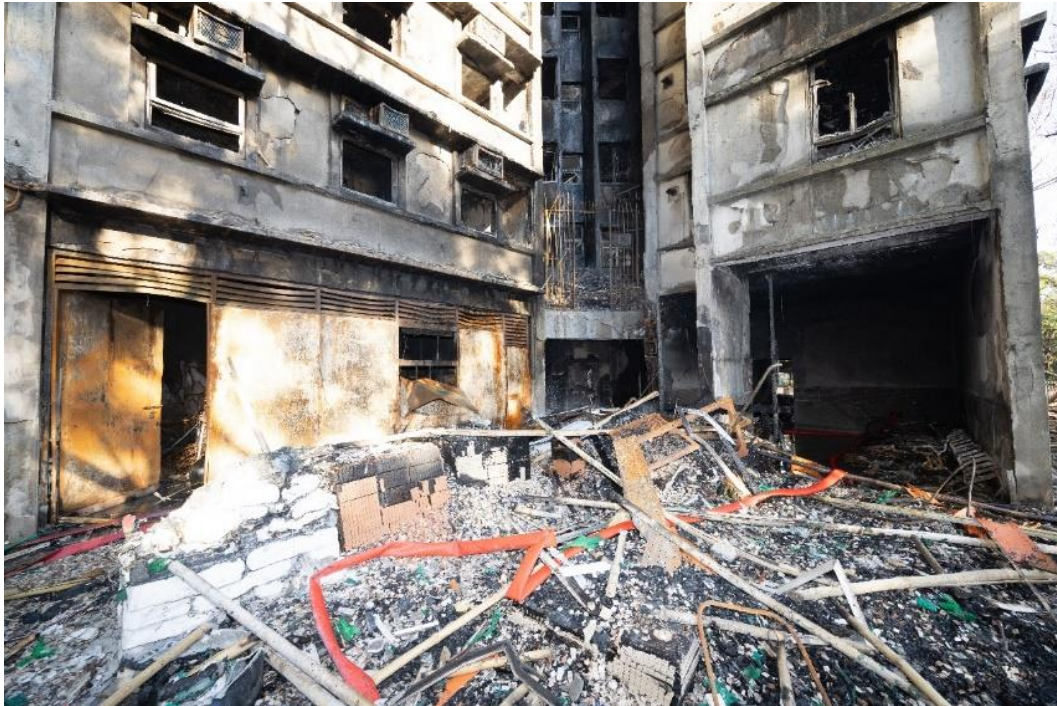
Photo 8-21 (g): Post-Fire Condition Outside the West Re-Entrant of Wang Tai House Facing Wang Kin House
