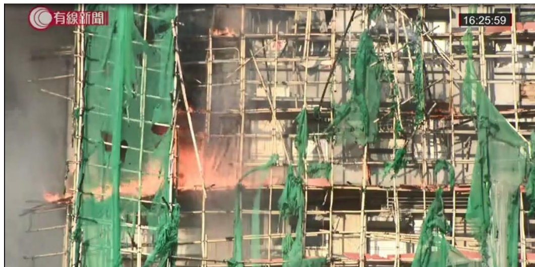
Photo 10-1 (c): Combustible Envelope Fueling Fire Spread
