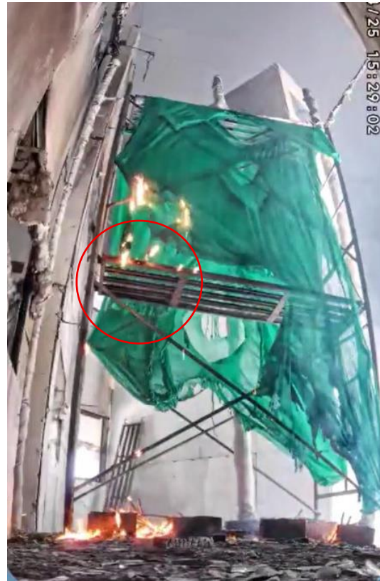
Photo 7-4 (c): Extensive Fire Spread on Sample 4 (Wang Chi House)
