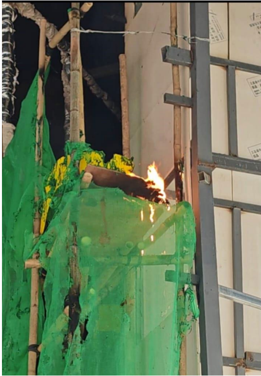
Photo 2-17 (e): Fire Spreading to Wooden Planks and Toe-Boards
