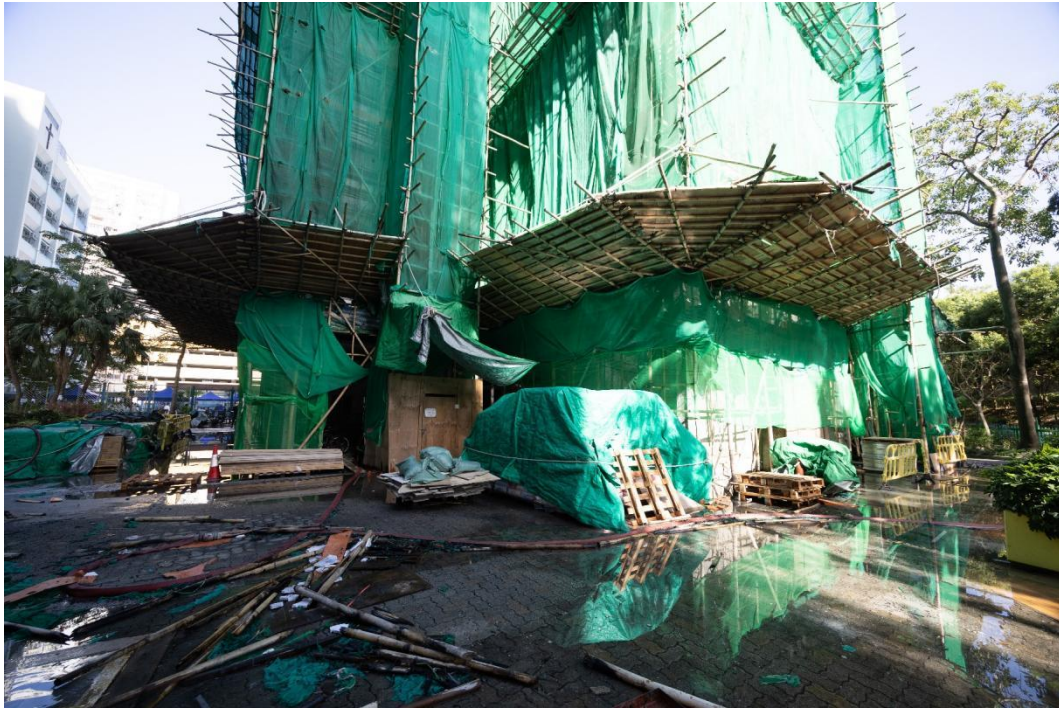
Photo 4-10: Construction Materials Scattered at Ground Level Around Wang Chi House
