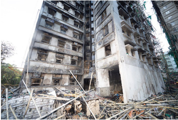
Photo 4-9 (a): Post-Fire Condition outside the East Re-entrant of Wang Cheong House
