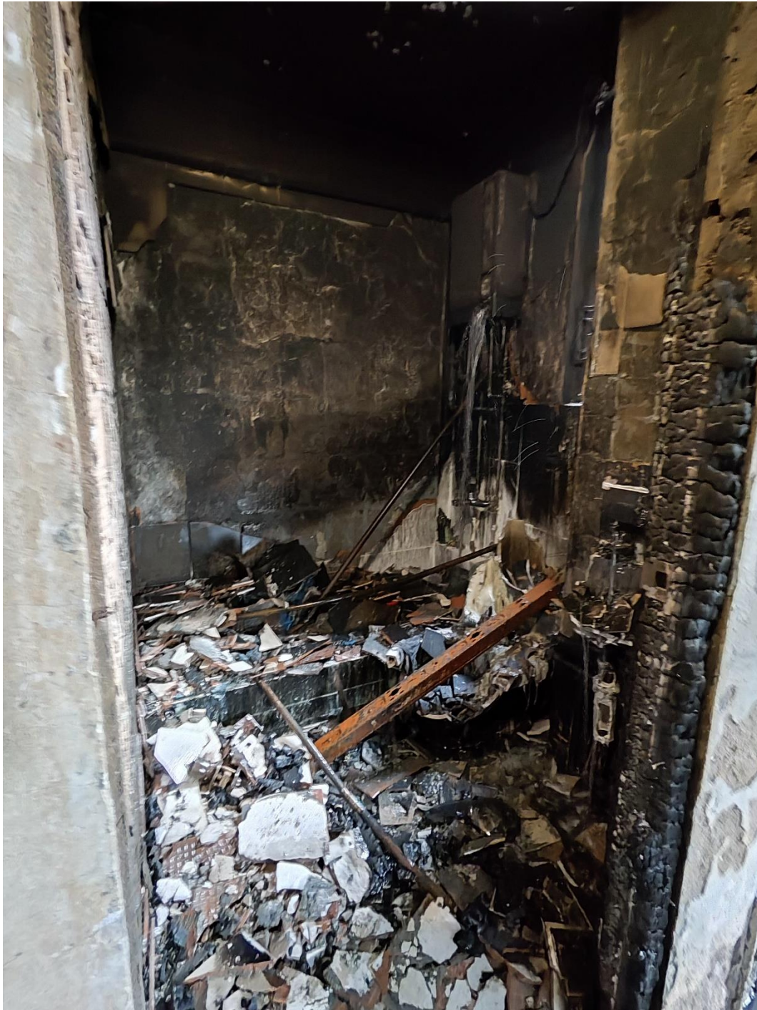
Photos 10-5 (a) to (f): Post-Fire Condition of Flat 2█, Wang Cheong House
