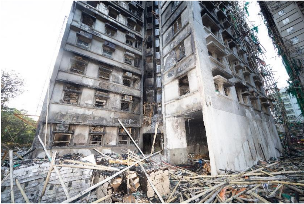
Photo 8-21 (a): Post-Fire Condition Outside the East Re-Entrant of Wang Cheong House
