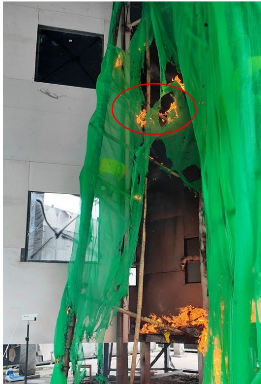
Photo 2-12 (f): Fire Spread to Other Construction Materials in Test 8
