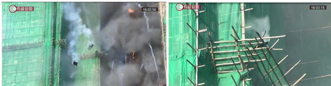
Photo 10-1 (b): Secondary Ignitions Caused by Falling Debris
