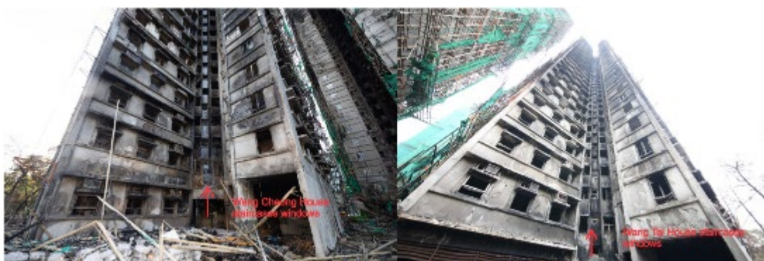
Photo: Most of staircases' windows of Wang Cheong House and Wang Tai House were damaged by fire.
