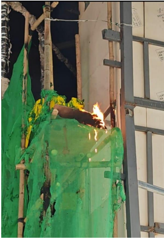
Photo 7-5 (e): Fire Spreading to Wooden Planks and Toe-Boards
