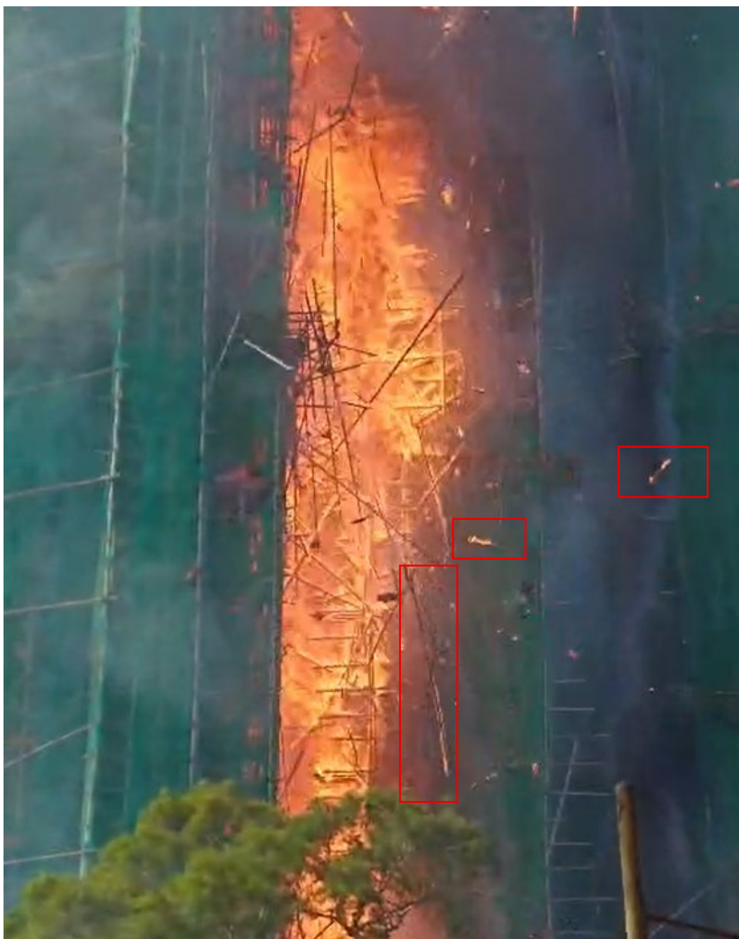
Photo 4-7: Collapsed Burning Debris from the Damaged Bamboo Scaffolding
