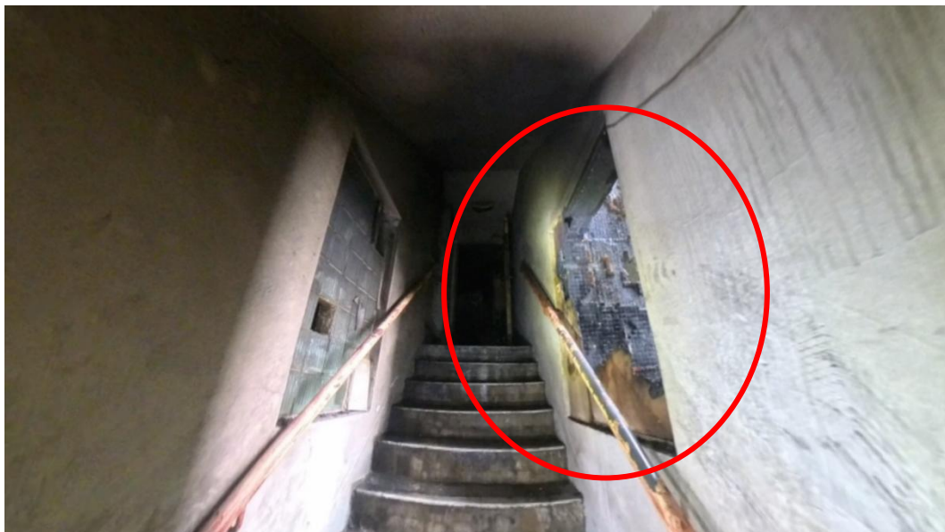
Photo 10-8 (a): Windows Replaced by Movable Boards (Damaged by Fire) at Escape Staircase of 10-11/F of Wang Tai House
