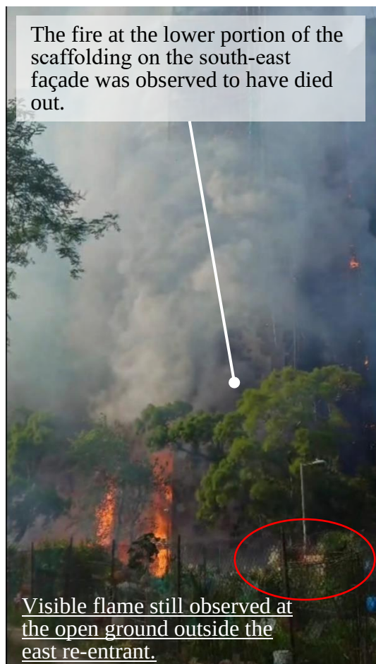
Photo 5-6 (d): Visible Flame Still Observed at the Open Ground outside the East Re-Entrant at 1508 Hours
