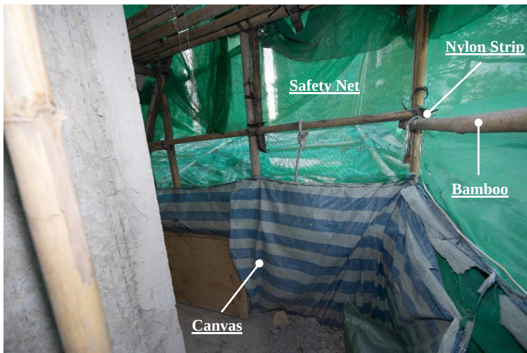
Photo 4-5: Photo Showing Different Combustibles in the Scaffolding (Bamboo, Safety Nets, Canvas and Nylon Strips)
