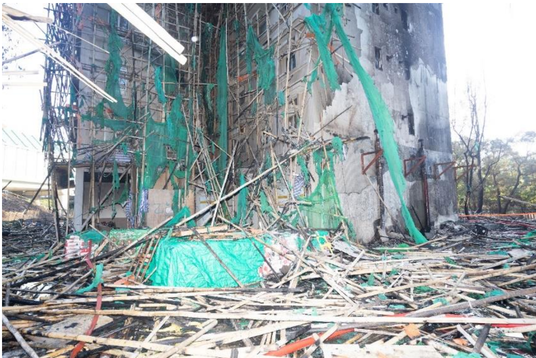
Photo 8-21 (h): Post-Fire Condition Outside the North Re-Entrant of Wang Cheong House
