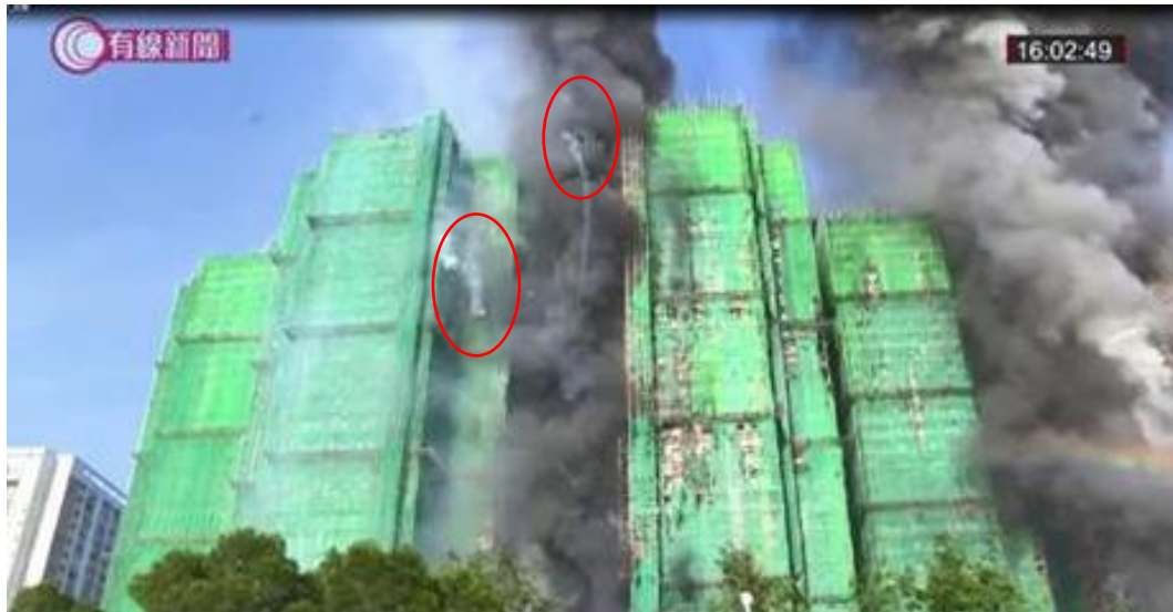
Photo 8-18 (a): Debris Falling From Wang Sun House at 1602 Hours
