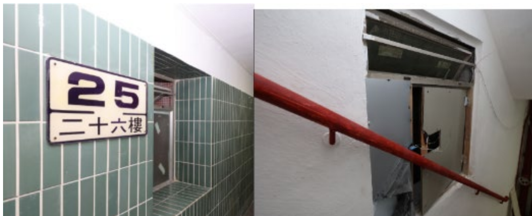
Photo: External windows at the staircase on twenty-fifth floor removed and replaced with wooden boards and locks.
