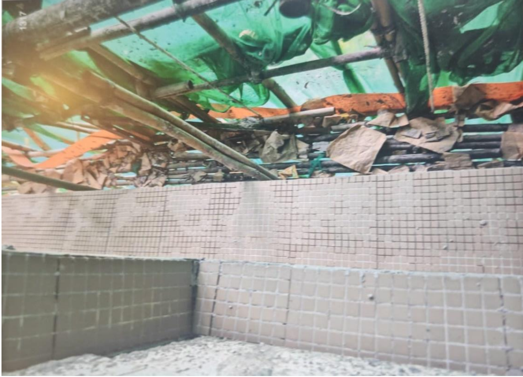
Photo 8-19 (c): Combustible Waste on the External Scaffolding
