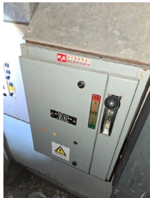
Isolator of Meter Room (Photo M2)
