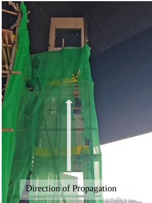
Photo 8-20 (a): Small Fire Propagated Along the Safety Net
